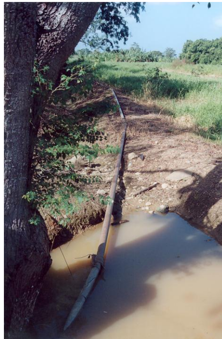
Figure 10: Galvanise conduit taking polluted water into production fields
